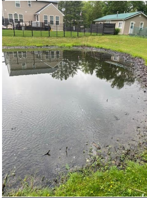
Figure 1. Aqua Doc Pond #13 (Herrington Pond #19) – Low water level; Recommendation to Dredge (boarding on Swamp conditions instead of Retention Pond Basin)
